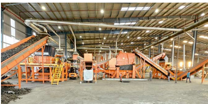
Fornnax OTR Tire Recycling Plant
