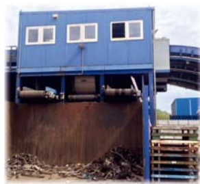
Ventilation & Venting for Sorting Cabins
